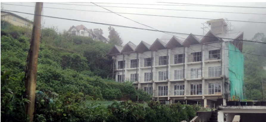
88 TH Developer (Pvt) Ltd-Nuwaraeliya Project (Supply & Installation of Total Fire Protection & Detection System)
